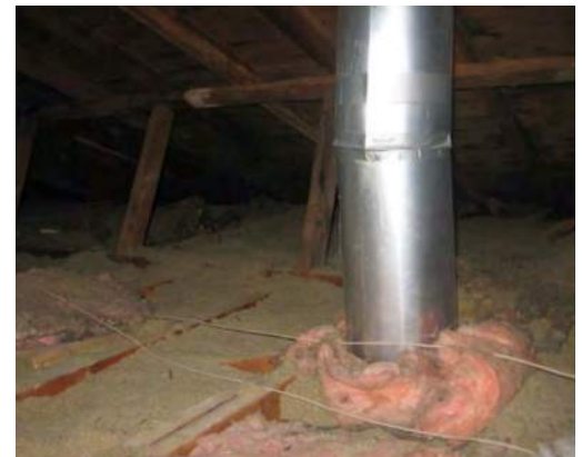
Insulated exhaust duct in attic.
